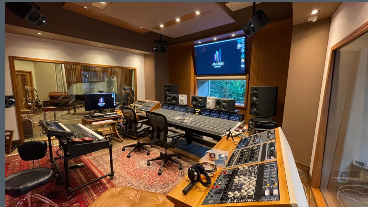
Dolby Atmos Control Room
