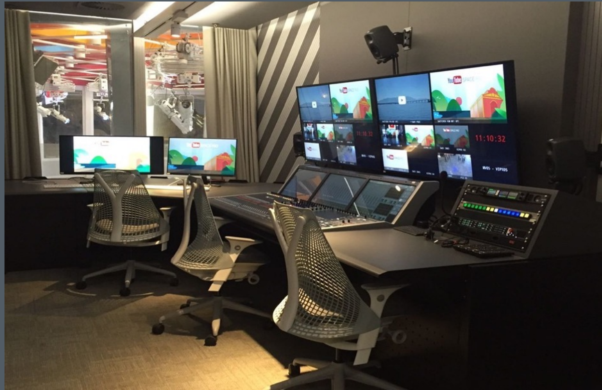
Audio Control Room
