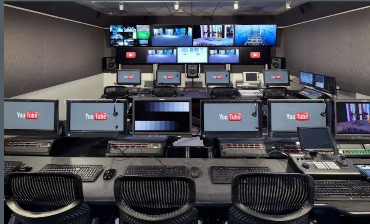
Video Control Room
