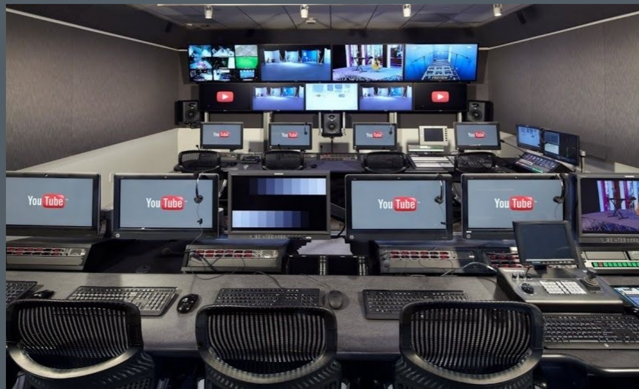
Video Control Room
