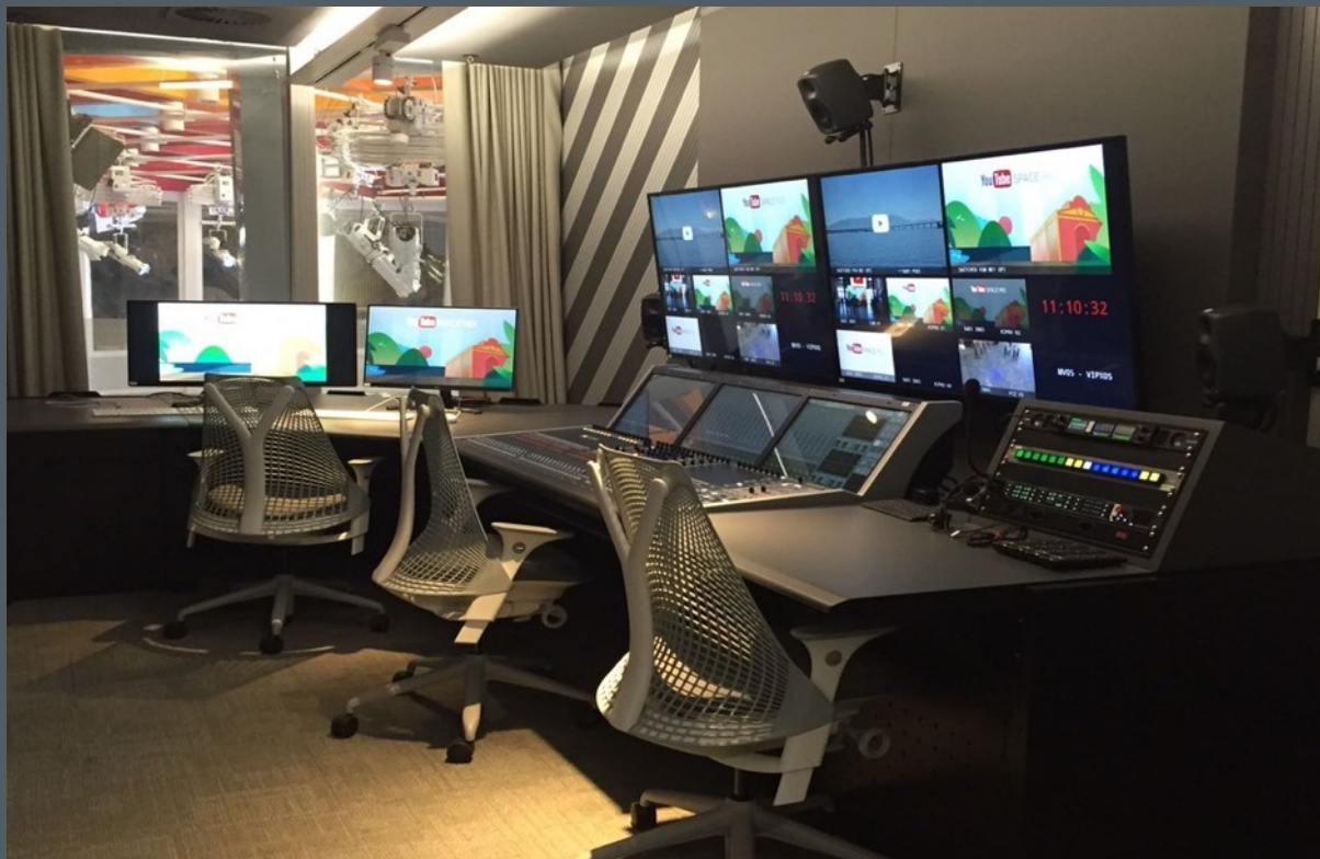
Audio Control Room
