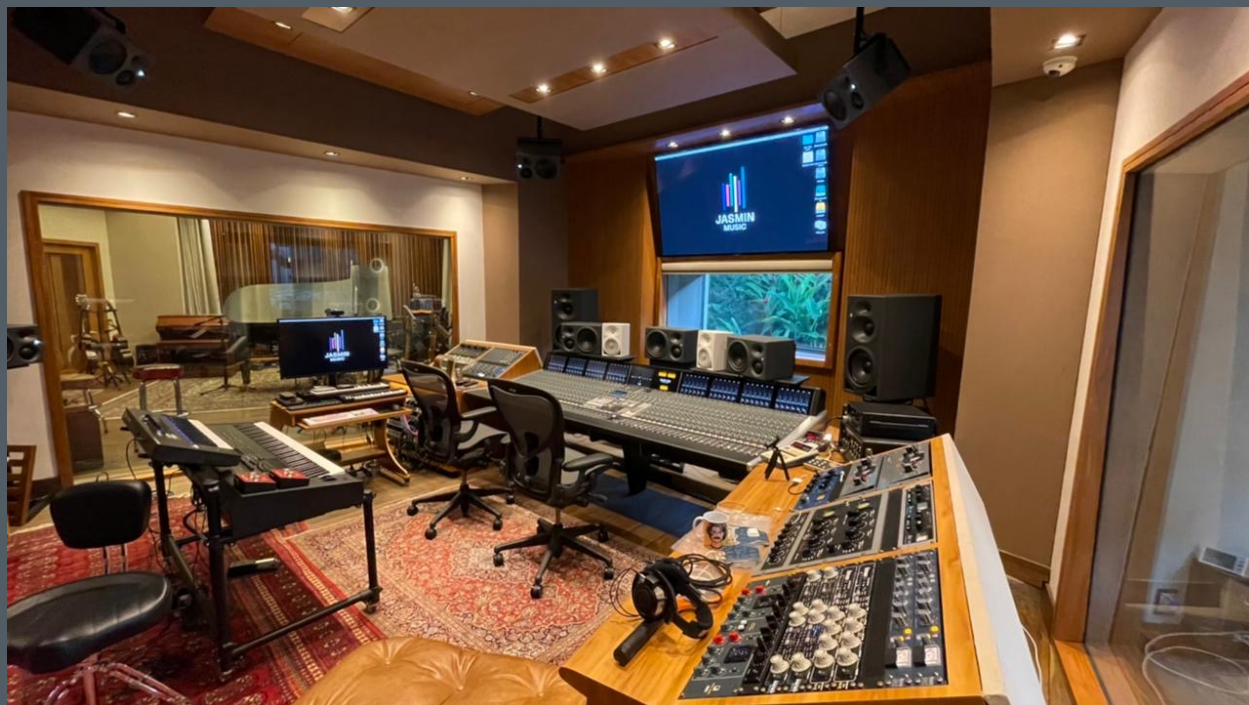
Dolby Atmos Control Room
