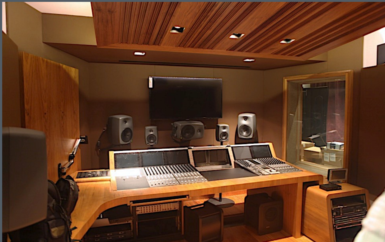
Audio Control Room
